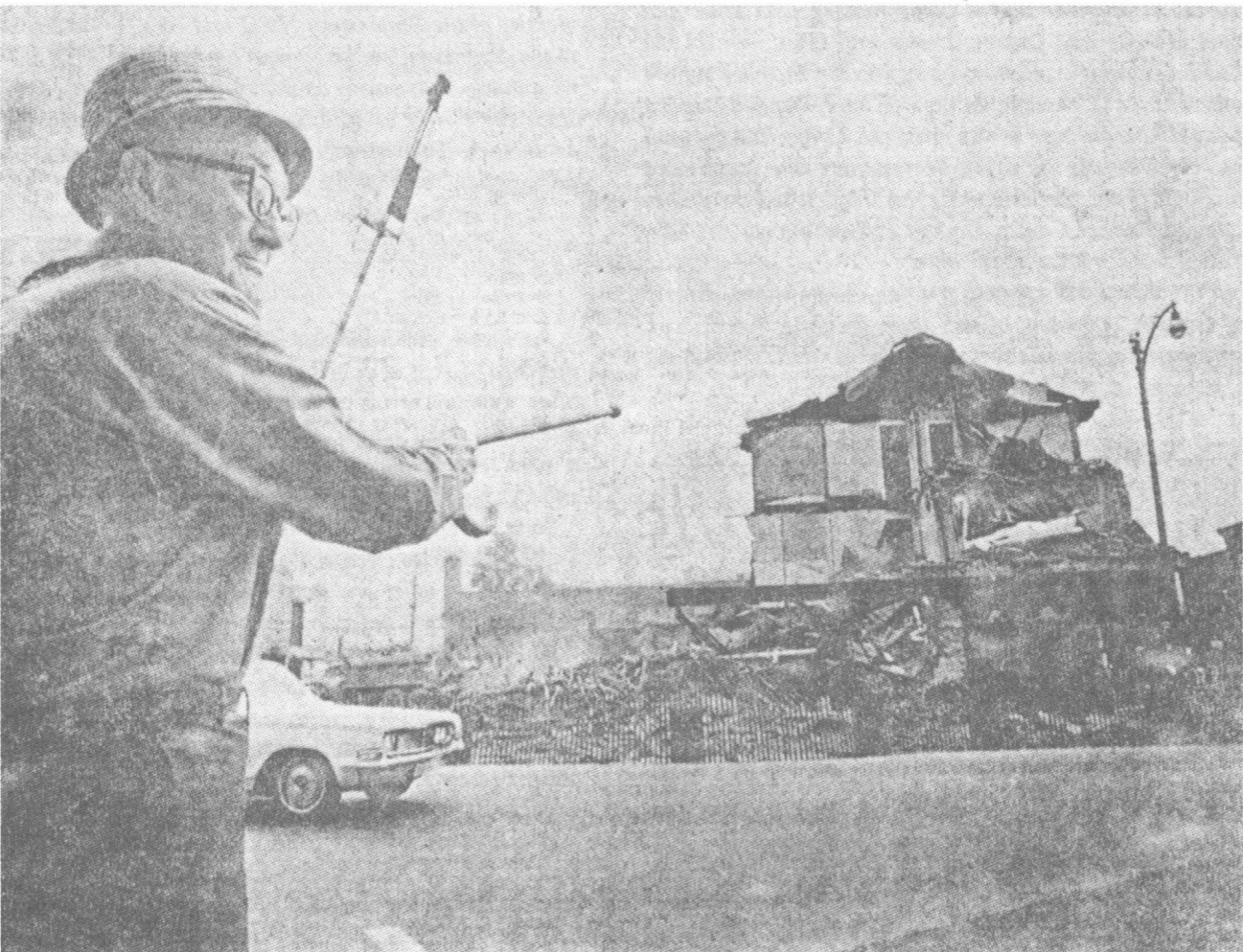
Frank Cleary watches the demolition of the Sinnissippi Hotel. After three years of public opposition, including a court case that reached the Illinois Supreme Court, the wooden-frame structure built in 1847 came down to be replaced by a gas station (Standard). (Photo courtesy of Republican Reporter)
