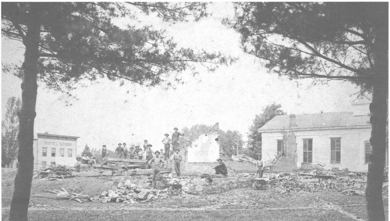
Razing of the second courthouse in 1890, to make way for the present courthouse. Note the old Lutheran Church to the right. (Courtesy of Mrs. Richard (Edith) Fridley)
