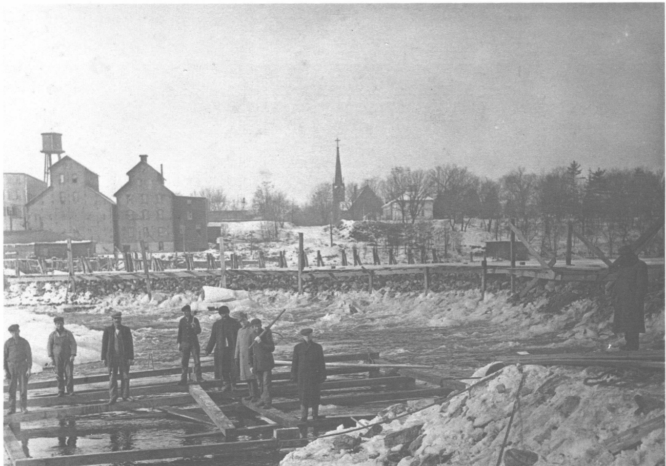
These men are building a crib which was sunk and filled with rock. The apron went over the top. Picture taken after 1906 while working on the dam. Note the timber hook over one man's shoulder. This kind of hook was also used on the railroads to carry ties. The buildings in the background from left to right are: Schiller, two Mills, Stan Jones house, St. Mary's church spire, old Conference Building of Church of God. (Photo courtesy E. G. Landers)
