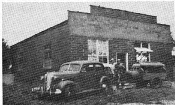
George Hedtke and Emil Svanda repairing the former Davis Junction Electric and Power Building 1943
